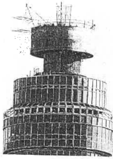
Raising a section of the steel tower by derrick pole at the top of London's Post Office tower.
